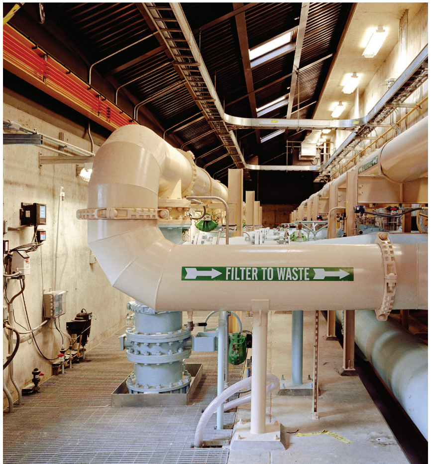
Additional filtration is sometimes employed by treatment plants that need to remove a greater level of solids from wastewater than is possible with standard methods. Plants may use this step or a combination of processes to meet the specific needs of their water.
