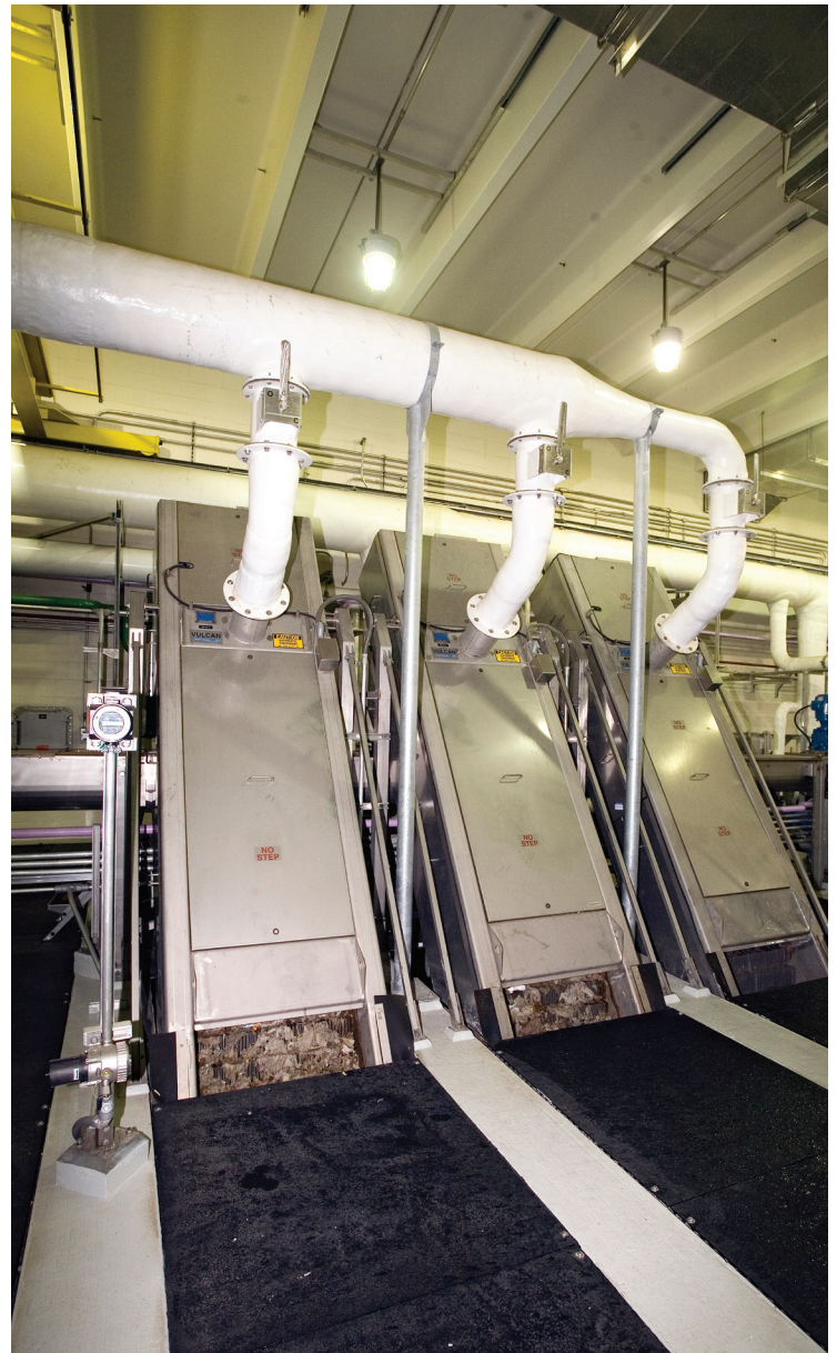
Large screens, like those shown here, are typically used to remove larger debris and other solid materials from wastewater as it enters a treatment plant.
