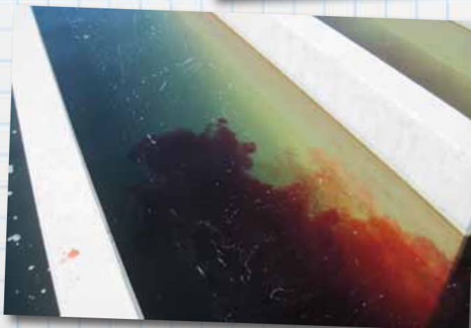
AFTER DYE TESTING AND CHLORINE RESIDUAL SAMPLES PROVE THE BAFFLES PROVIDE BETTER MIXING, THE TEMPORARY STAINLESS STEEL ANGLE BRACKETS AND 2X4 LUMBER BAFFLES WILL BE REPLACED WITH MORE ROBUST, PERMANENT MATERIALS.
