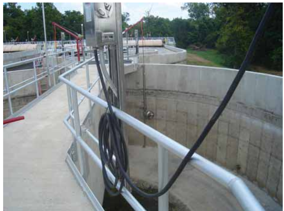
Maximizing the use of existing wastewater treatment structures is a consideration when addressing phosphorus requirements. In Salem, Ill., an existing tank was elevated and repurposed as an anaerobic reactor. CMT
