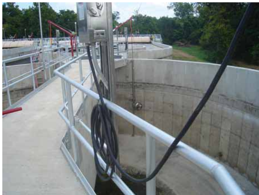
Maximizing the use of existing wastewater treatment structures is a consideration when addressing phosphorus requirements. In Salem, Ill., an existing tank was elevated and repurposed as an anaerobic reactor. CMT
