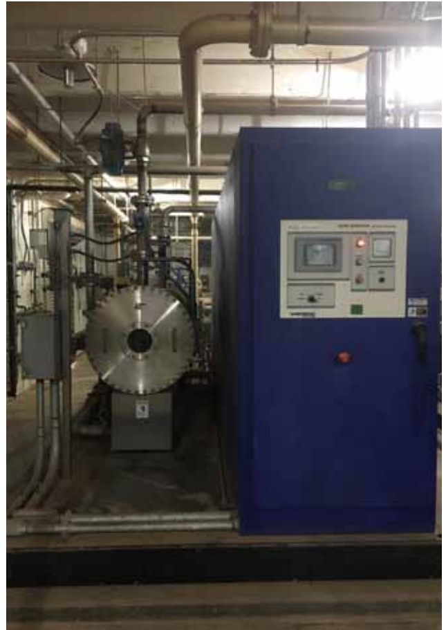
During the treatment, ozone is added to the treated water as the second step of the disinfection process for removal of viral and cyst organisms. The facility generates its ozone onsite. The action of ozone also breaks down organic material in the water improving the color, taste, and odor of the treated water. El Paso Water
