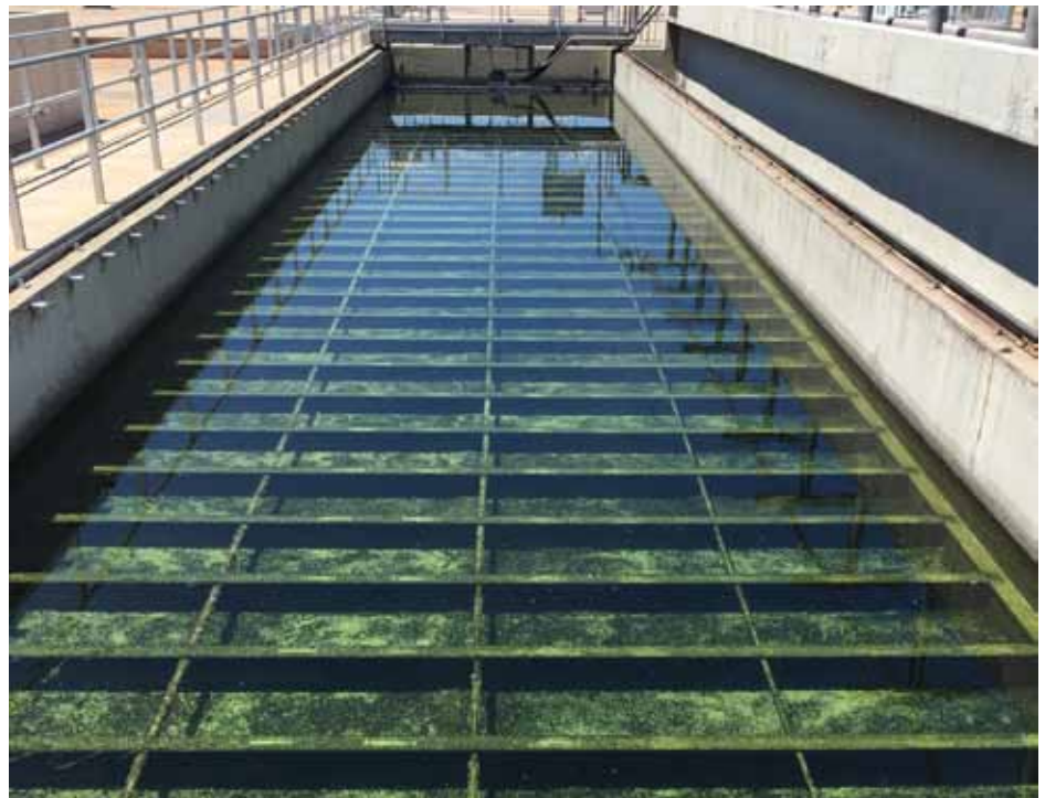
The sand filter removes light chemical flock from the effluent discharged from the second stage re-carbonation basins. This allows more effective contact of ozone with the pathogenic organisms and other oxidizable materials in the treated water. El Paso Water
