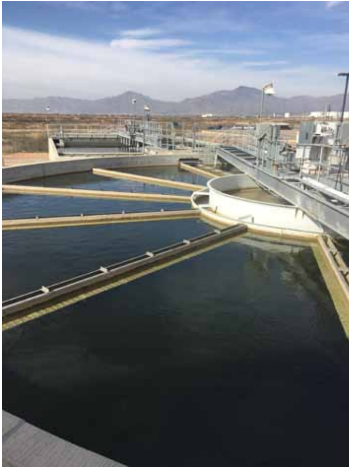
As the first step in disinfection, the lime reactor mixes a high dose of lime to the treated water to raise the pH, kill viruses, and remove hardness, phosphorus, and heavy metals. Carbon dioxide is then added to lower the pH. El Paso Water
