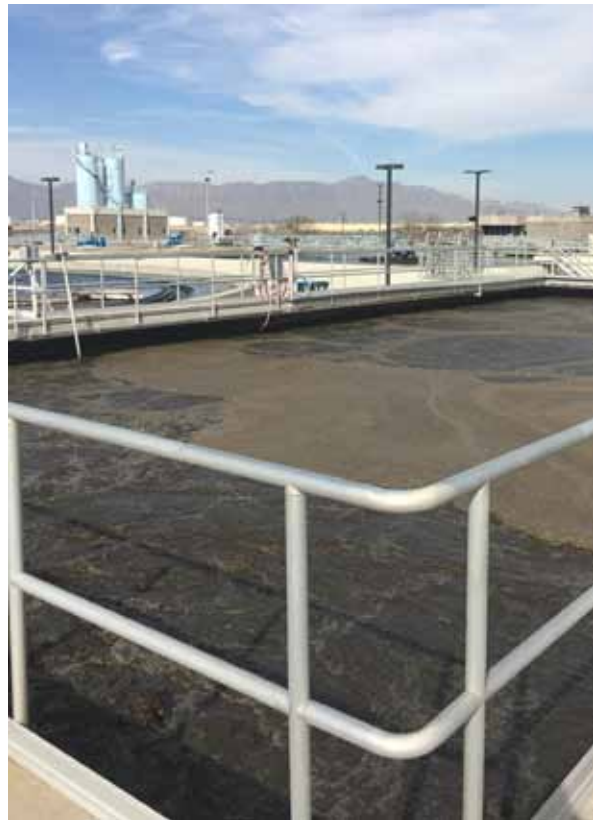
The aeration basin tanks provide an environment where activated sludge organisms consume and remove suspended organic matter while added PAC adsorbs pollutants. El Paso Water
