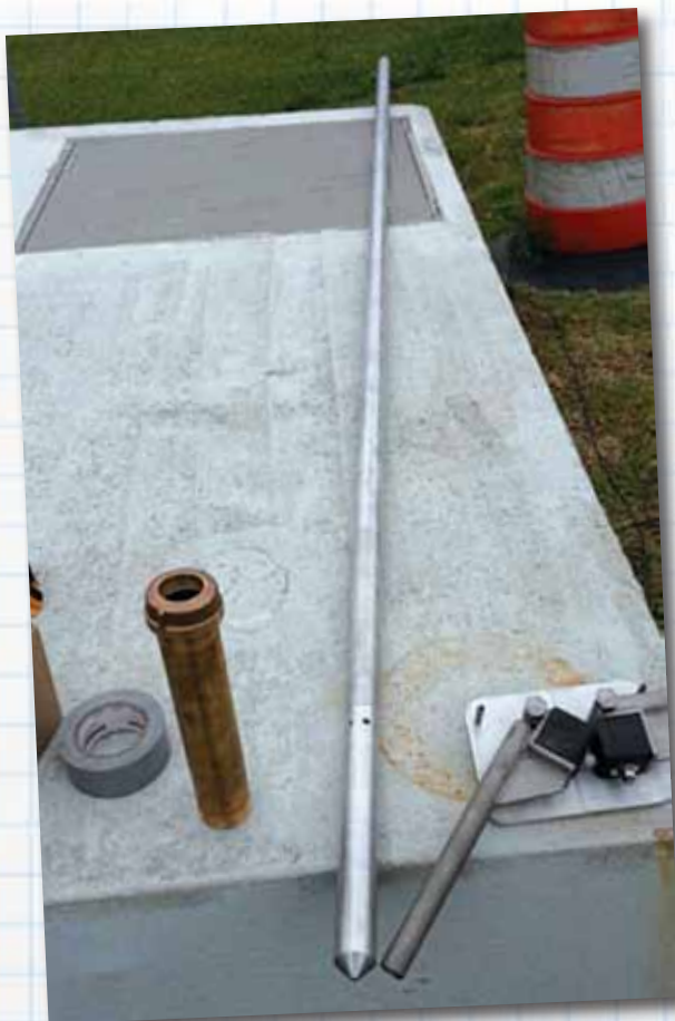
THE LONG RISER PIPE HAS A TAPERED END TO MAKE INSERTION EASIER. THE RISER COUPLING (COPPER PIPE AT LEFT) ATTACHED TO THE FORCE MAIN AIR RELEASE VALVE. THE HANDLE ASSEMBLY (RIGHT) ENABLED THE OPERATOR TO GRIP THE RISER PIPE AS IT IS SHOVED INTO THE FORCE MAIN. AN OPTICAL DISSOLVED OXYGEN PROBE IS INSIDE THE RISER PIPE. THE HOLES PARTWAY UP ALLOW THE WASTEWATER TO CONTACT THE PROBE WHILE PROTECTING IT FROM DEBRIS IN THE LINE.
