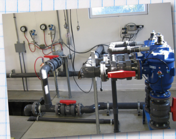
THE CITY OF AMES WATER POLLUTION CONTROL PLANT IN IOWA MOVED ITS EFFLUENT REUSE PUMPS INTO THE SAME BUILDING AS ITS NEW ULTRAVIOLET DISINFECTION SYSTEM. THE FILTERS, BACKWASH, AND PRESSURE CONTROL SYSTEM USE PRESSURE SENSORS TO RELAY INFO TO THE VARIABLE SPEED DRIVE CONTROL FOR THE PUMPS TO MAINTAIN A CONSTANT PRESSURE AND PUMPING CAPACITY.
