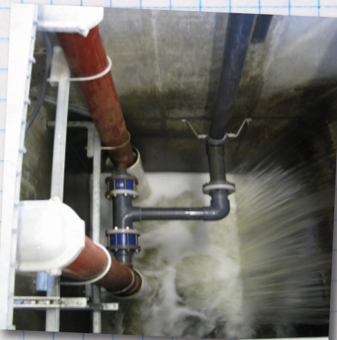
THE BROWN PUMP CASINGS EXTEND INTO THE WET WELL IMMEDIATELY BELOW THE ULTRAVIOLET DOSAGE CONTROL GATE. HOWEVER, THE TURBULENCE OF THE WATER CAUSED CAVITATION IN THE PUMPS, RENDERING THEM UNUSABLE.
