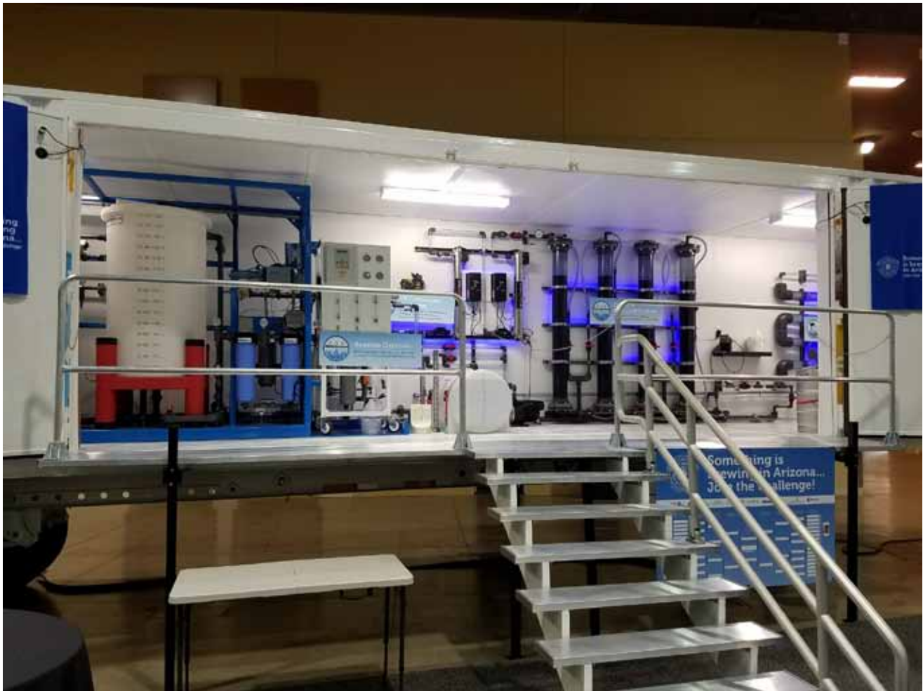
The interior of the AZ PURE Water advanced purification facility was designed to be clean and sterile to reinforce a sense of quality. It provides an excellent background to highlight the treatment technologies being used in the project. Pima County
