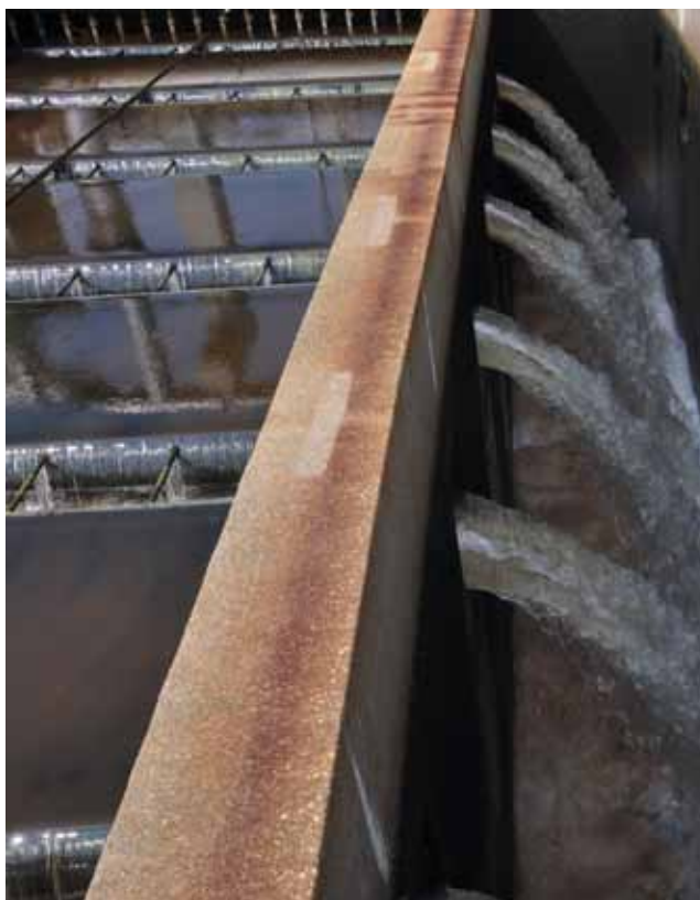
In 1982, the Blue Plains Advanced Wastewater Treatment Plant in Washington, D.C., added multimedia filtration following advanced nutrient removal. These filters remove additional suspended solids and associated phosphorus. DC Water
