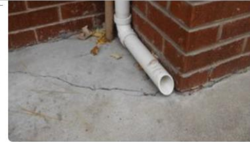
Discharge - Storm Sump
