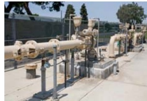
Typical injection well - OCWD
