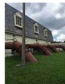
Photograph 32: PS 536 Side with discharge suction piping
