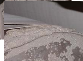
Deposits on belt filter press rollers
