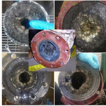
Deposits in pipes
