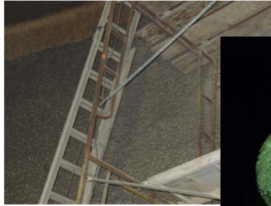
Deposits on digester wall
