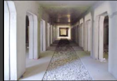
Underground infiltration chambers at
