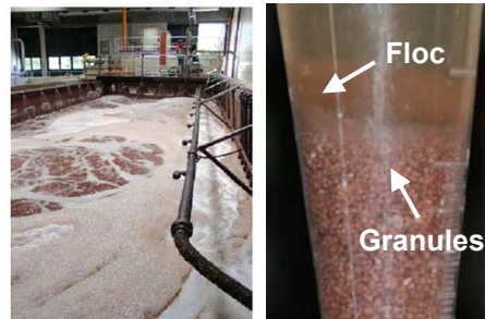
DEMON® Reactor at Strass WWTP
