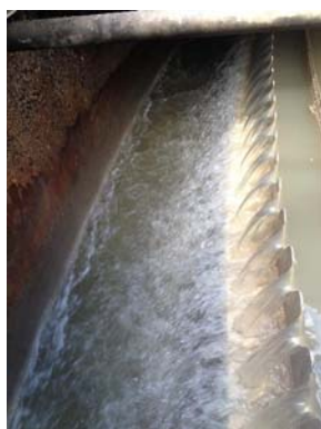
Primary Weir Drop
