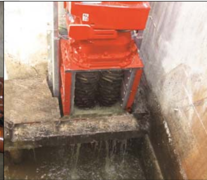
Raw Sewage Channel
