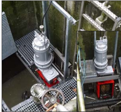
Wet Well Grinder
