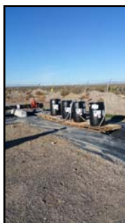
Granular Activated Carbon Drums
