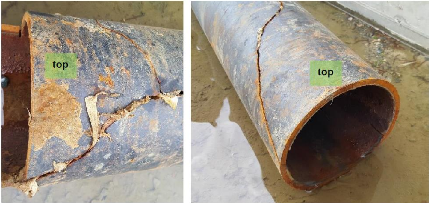
Figure 9: Wayne Creek watershed site map used for assisting in location of contamination sources – photographs of the resulting identified cracked pipe as the source.
