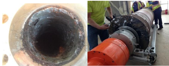
Figure 1: Vivianite Scale Formation in (a) Flow Meter Pipe and (b) Centrifuge Dam Plates
