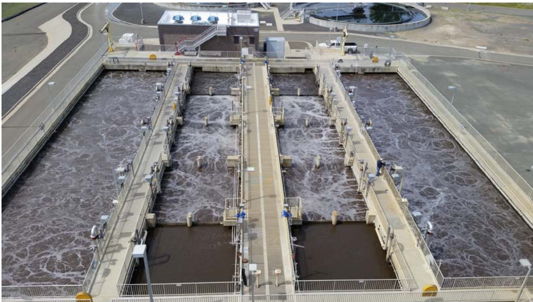
Figure 1— Fine Bubble Diffused Aeration System in Action. Photo courtesy of Napa Sanitation District.
