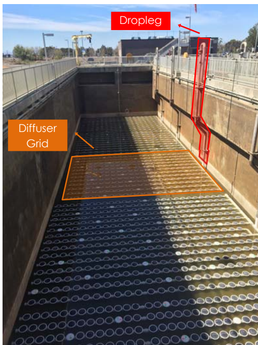
Figure 2— Droplegs and disc diffuser grids. Photo courtesy of Napa Sanitation District.
