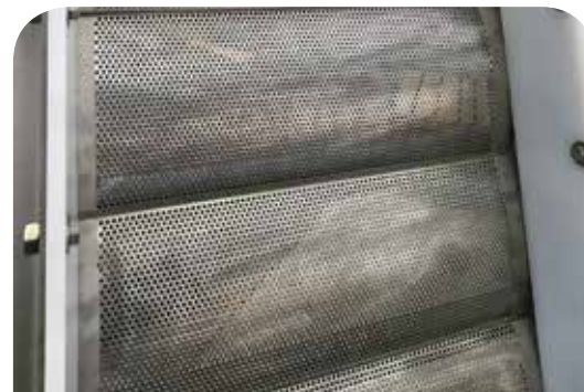
Mexico Perforator® 2 units, 6.5 feet wide 34 MGD each (128 MLD)
