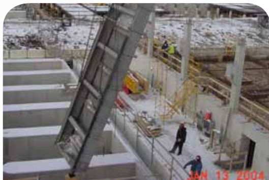
USA, Michigan MS™ Bar Screen 16 units, 10 feet wide 5,940 MGD (22,485 MLD)
