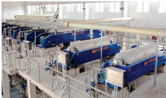
DingFuZhuang WWTP Beijing, China: Five Centrisys THK600 and four CS21-4HC.
