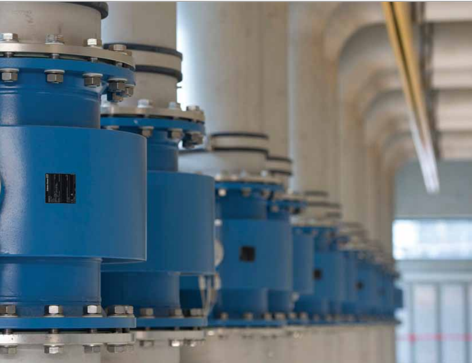
Flow measurement of water, wastewater or sludge: The electromagnetic induction method of flow measurement is the standard
