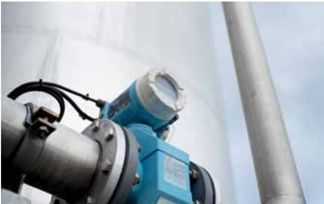
Industrial water treatment and wastewater treatment
