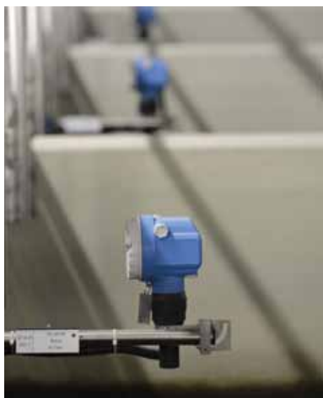
Reliable level monitoring of basins
