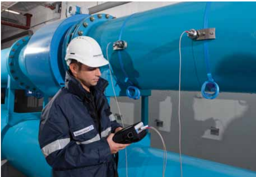
Verification of a flow measurement during live operation by an experienced service technician
