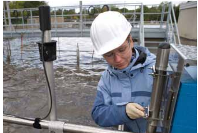
Our experts provide on-site support for smooth plant operation
