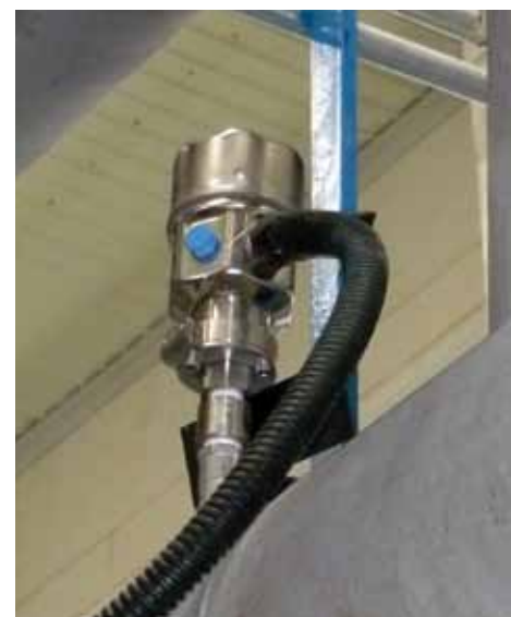
Accurate pressure measurement in a membrane system
