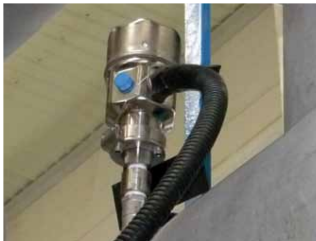
Reliable pressure measurement in a membrane system
