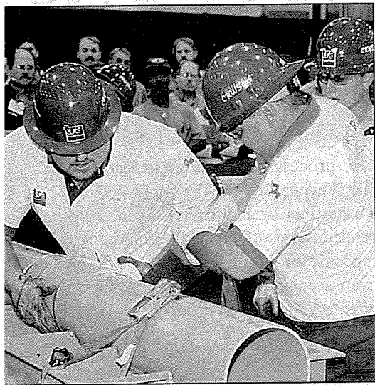
John Bennet (left) and Steve Price (right) of Team TRA CRWSers (Texas Water Environment Association) cut and prepare a repair piece for a PVC pipe in the Collections event, placing third overall in Division 1.
