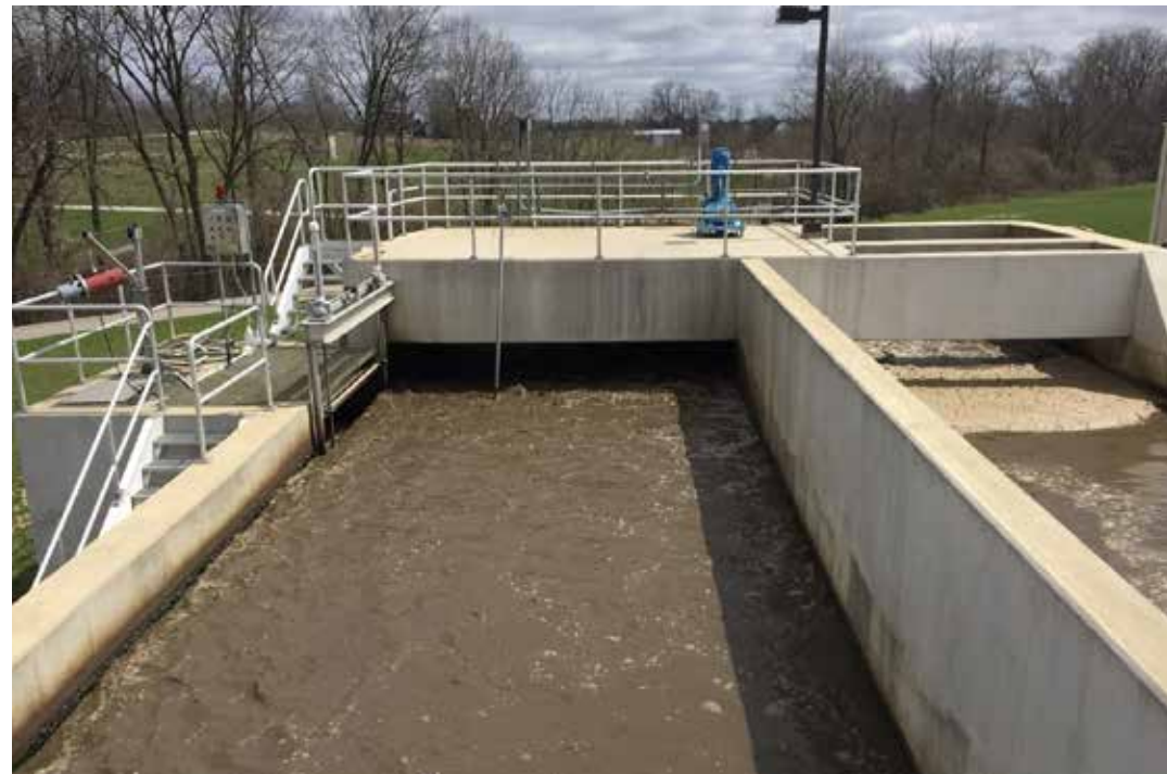
The rotor in this tank was run at minimum hertz to gain simultaneous denitrification on the back side of the oxidation ditch. Jon van Dommelen
